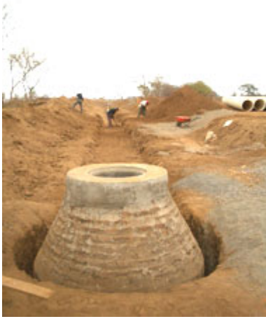
Waste water system
